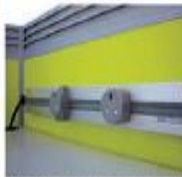
External Console of switch, power point, telephone point and data point.
